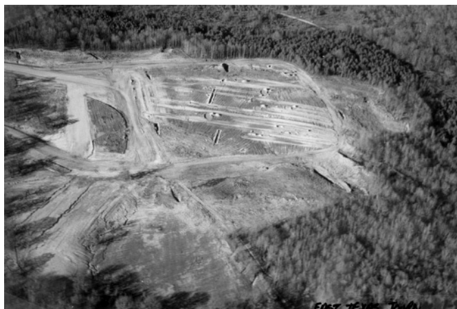
Figure 1-2. Aerial overview of the Pilgrim's Pride site, with access roads encircling the site, and trenches and road grader scrapes excavated by Keller visible throughout the site.
