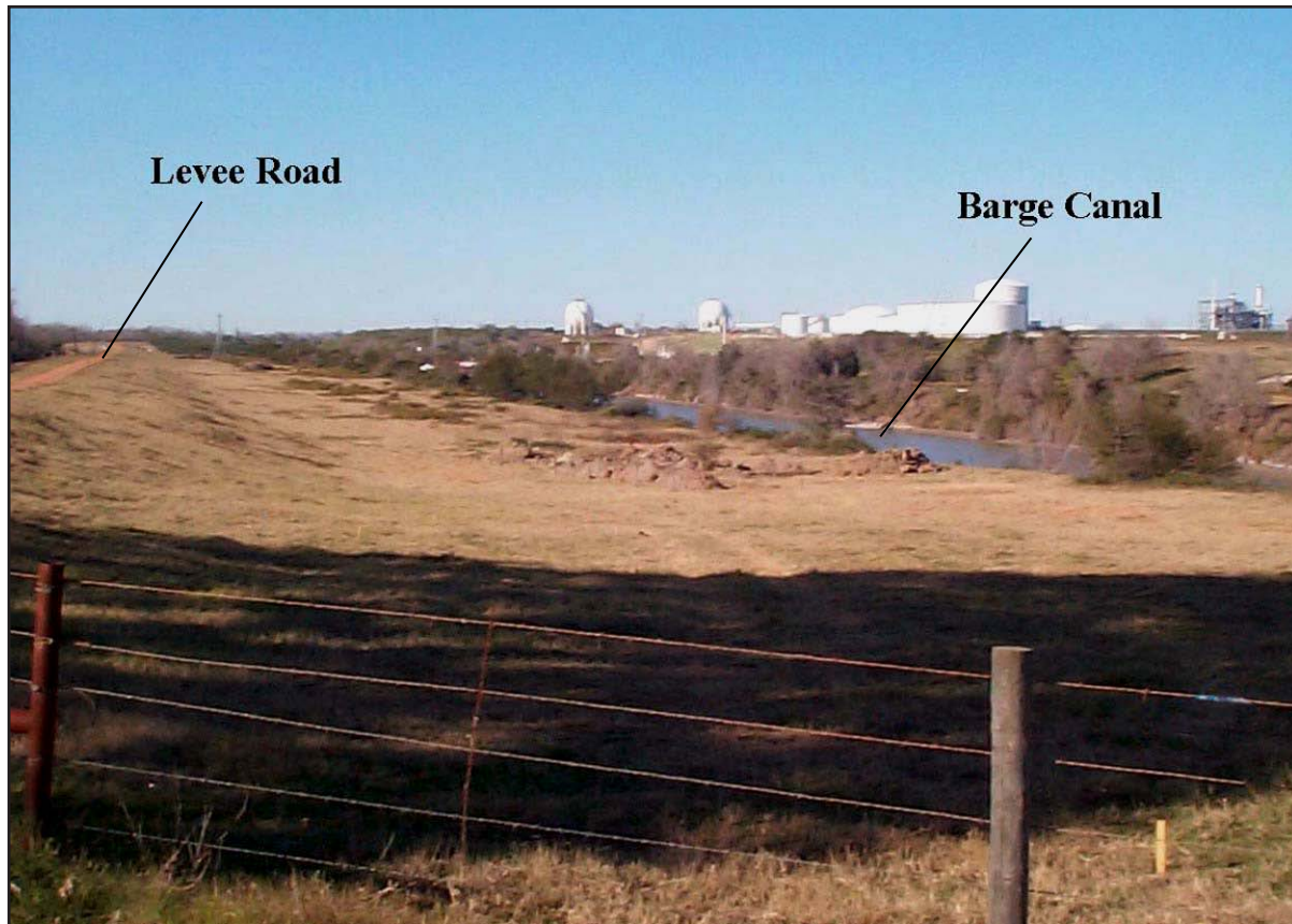
Figure 3-2. View of the West Canal Bank Area at the Buckeye Knoll site looking northwest and showing backhoe trenches during excavation.
