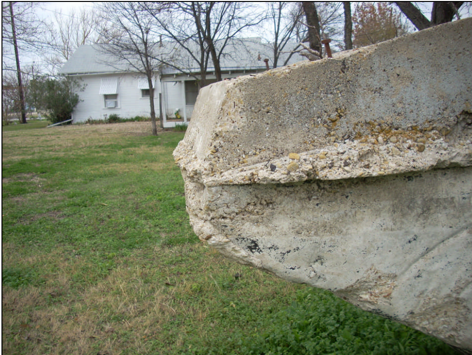
Figure 4. Profile of the entrance to storm cellar. Note the amount of concrete on the side of the entrance.
